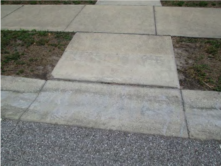
Missing ADA Ramp east side of Honeyflower Loop
