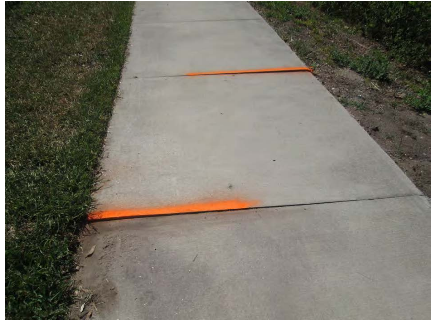
Grinds at lot 268 Chantilly Trail
